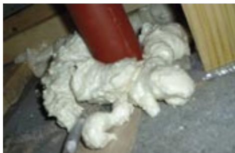
Figure 16 Poor sealing around a service pipe.
