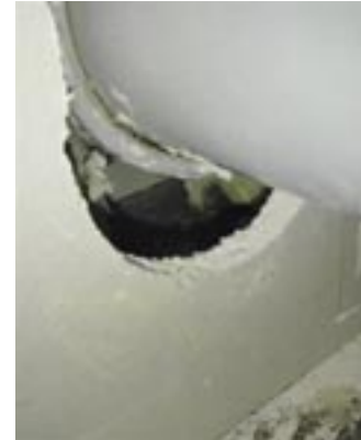
Figure 3 Gap around soil pipe at back of toilet.
