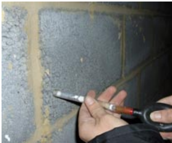
Figure 4 Air permeability through gaps in a blockwork wall.
