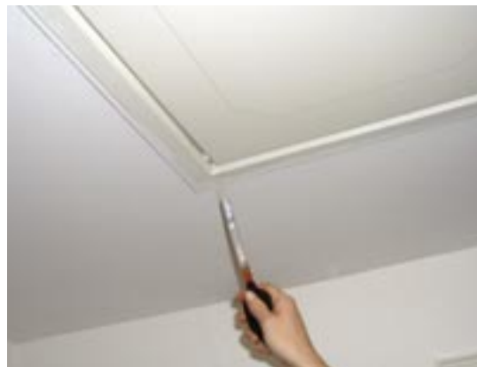
Figure 2 Air leakage through gaps around a loft hatch.
